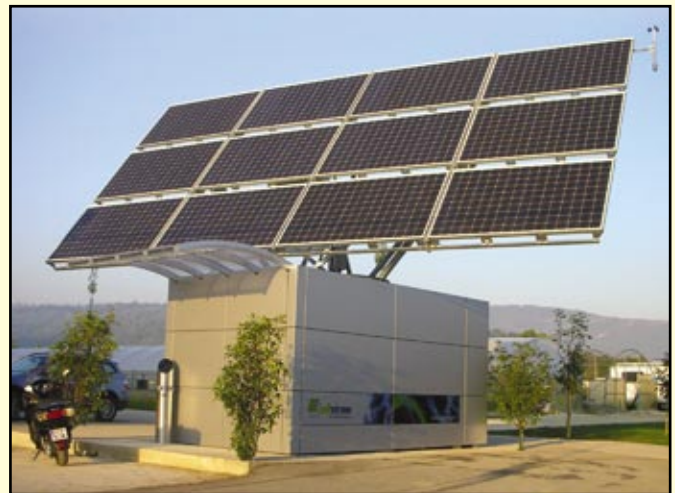
A Vanadium battery powers a solar charging station for electric vehicles at a wine and olive farm in Perugia, Italy.
